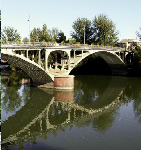
The assembly of the three-point arches, together with the use of reinforced concrete, enabled the construction of the Pont Neuf to include extremely delicate features and a markedly hollowed structure.
